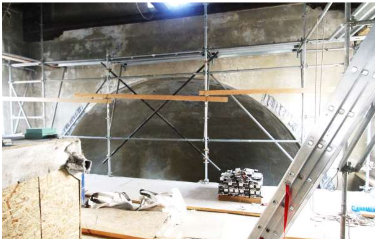
The internal plastering surfaces before restoration
