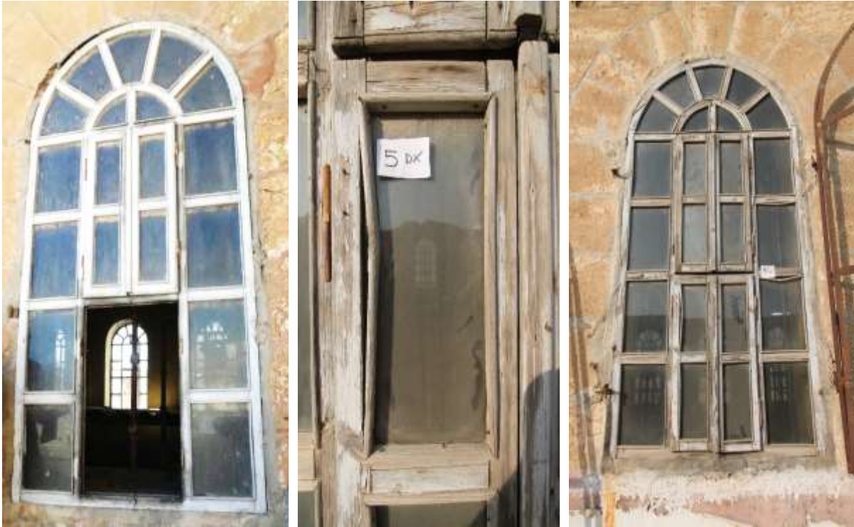
The damaged wooden windows
